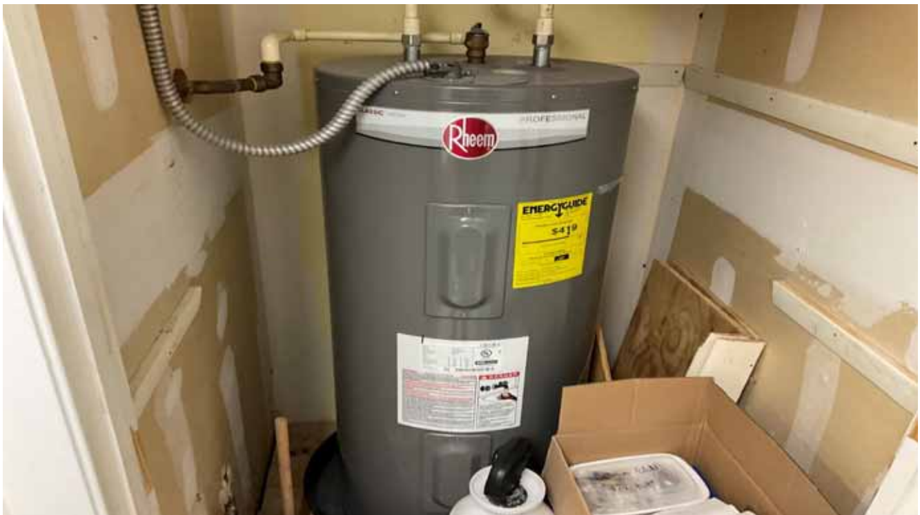
Water Heater - Restrooms
