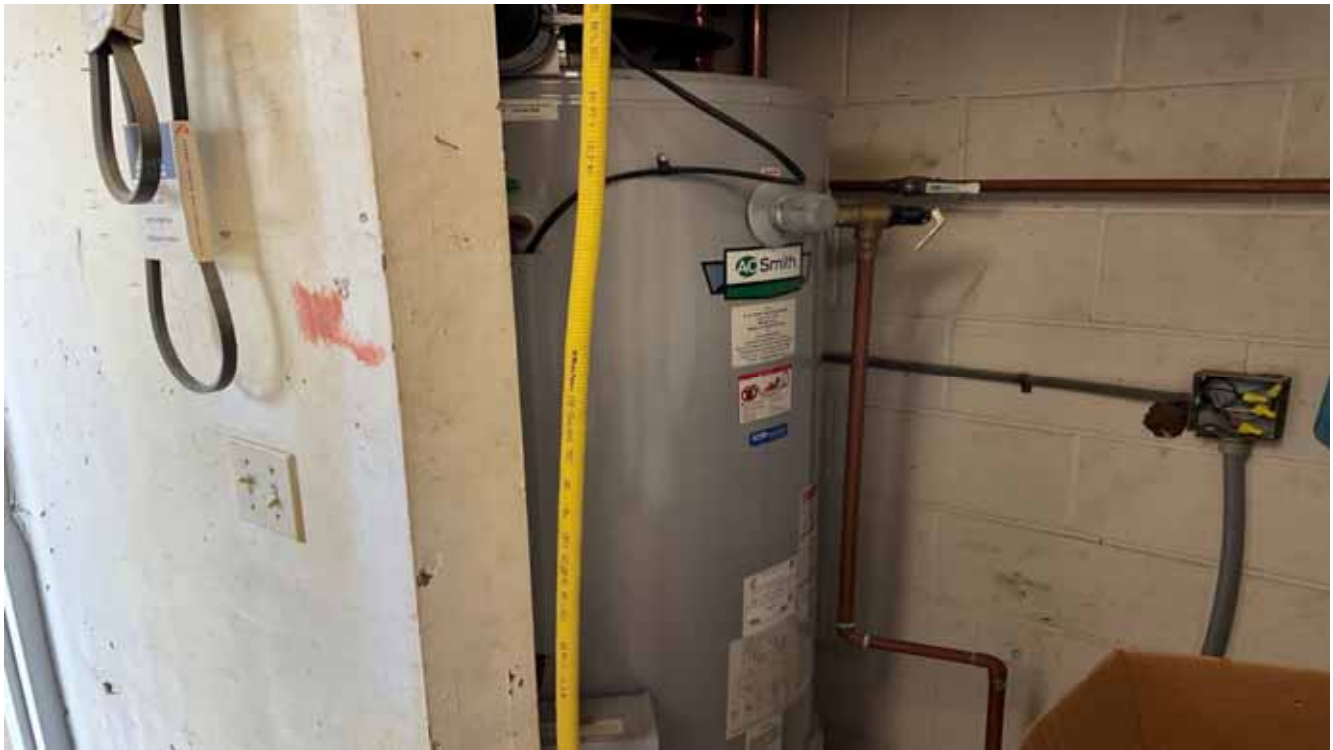
Water Heater - Kitchen
