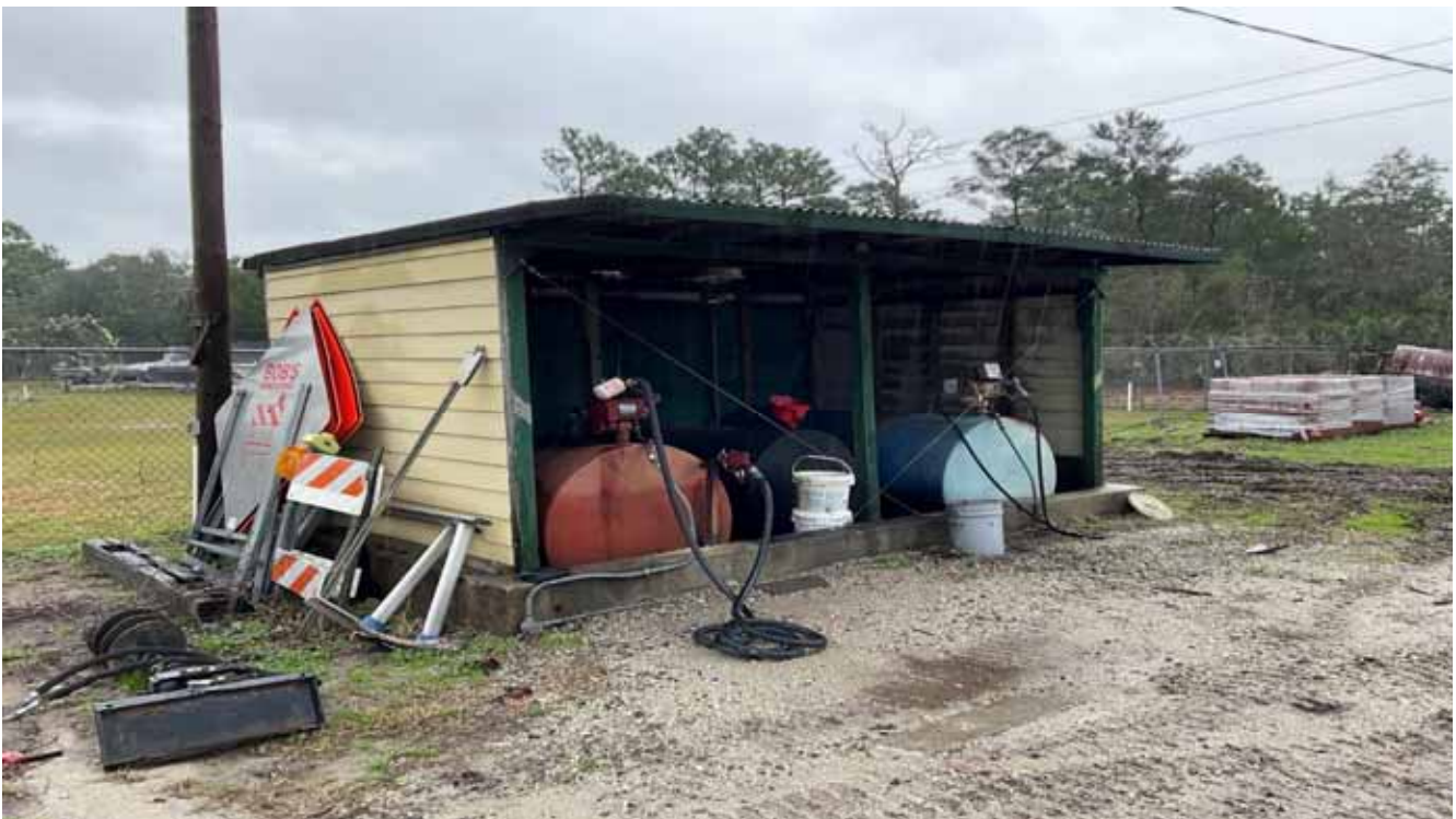
Maintenance Fuel & Oil Tanks
