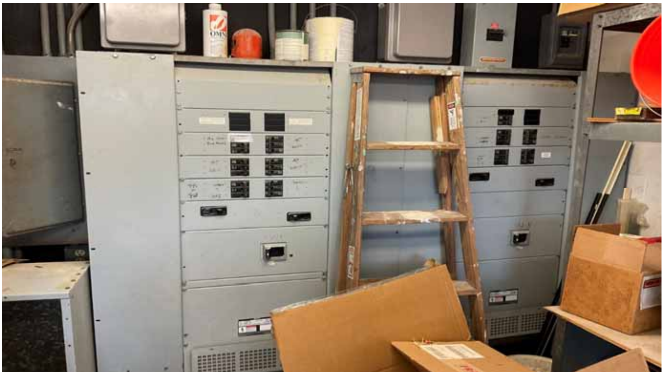
Main Electrical Room
