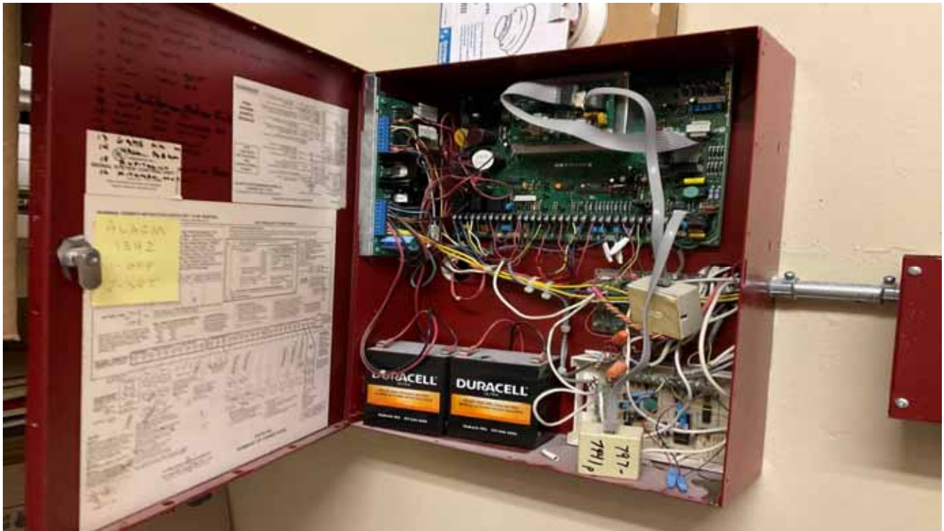
Fire Alarm Control Panel
